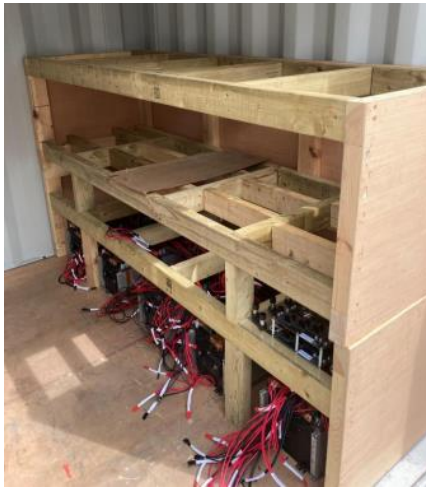
Stationary energy storage
